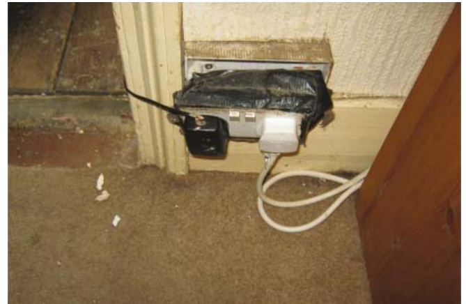
Figure 2: Property 2 showing a dangerous electrical socket with a high risk of electrocution
