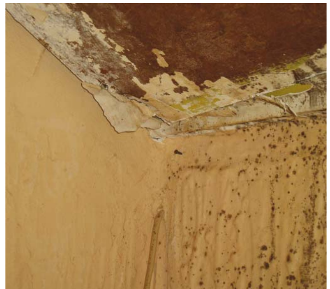
Figure 3: Property 3 showing damp and mould growth in the single storey extension
