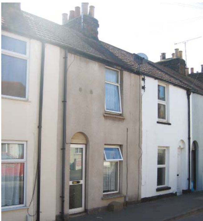
Figure 1: Property 1 showing an open low sill window vent on the first floor, with a high risk of fall
