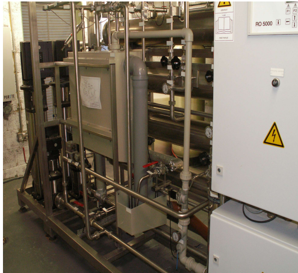
The reverse osmosis system in the Ashford Satellite Dialysis Unit.
